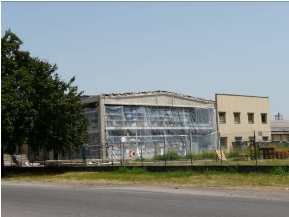
Fig. 40. View of prefabricated building with collapses on façade elements (Mirandola)
