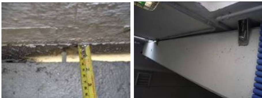
Sports hall Magnani – (general view and details of the weak supports)
