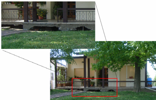
Fig. 18. Settlement of shallow foundation of a cottage because of liquefaction (S. Carlo).
