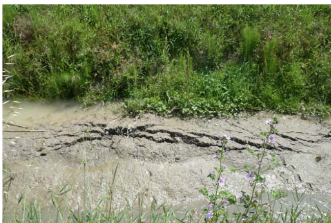
Fig. 27 – Uccivello di Cavezzo: bed of a canal uplifted, bulged and cracked due to sand ejection from beneath its bottom after the 29 th May earthquake.
